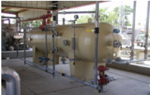
Water Phase Equipment
